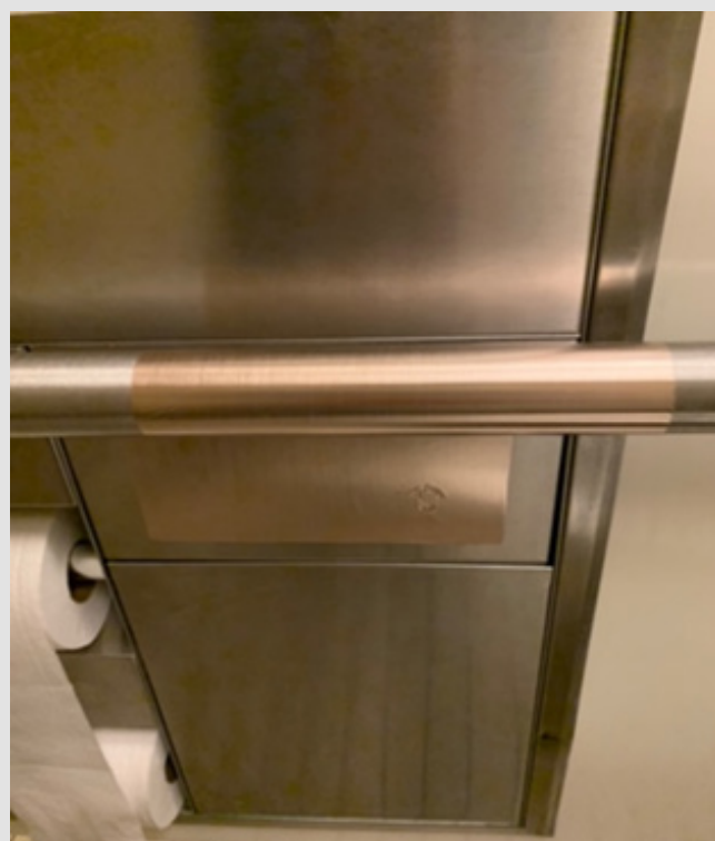
Figure 1: Antimicrobial copper on LA MTA bathroom handicap grab rail and trash receptacle door.
