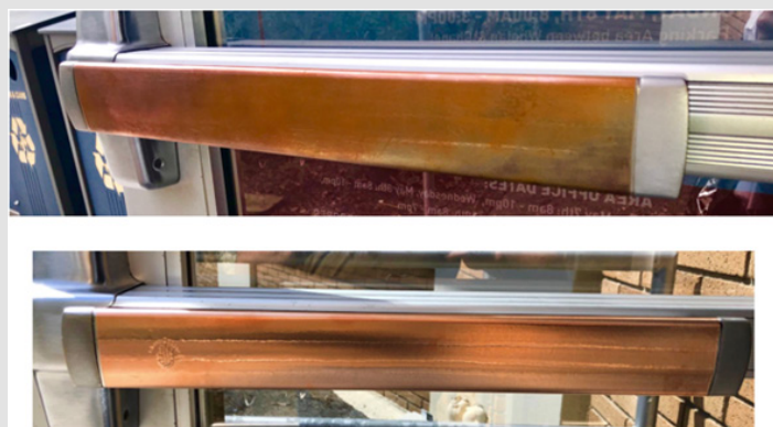
Figure 2: Front entrance push bar handle. A. Immediately upon installation. B. 1 month after.
