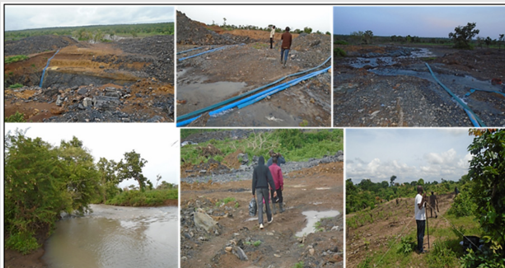
Plate 2: Mining Sites Characterized by Vegetation and Water Bodies. Hosepipes laid in mining pits for discharge of water into flowing water bodies around.
